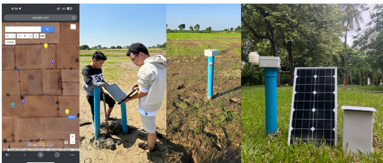
Figure 29: Field Test of Automatic Water Monitoring Device (2nd Prototype)
